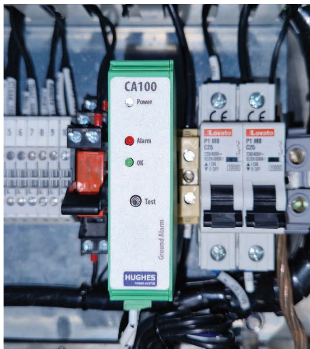
Installation in the motor drive cabinet
